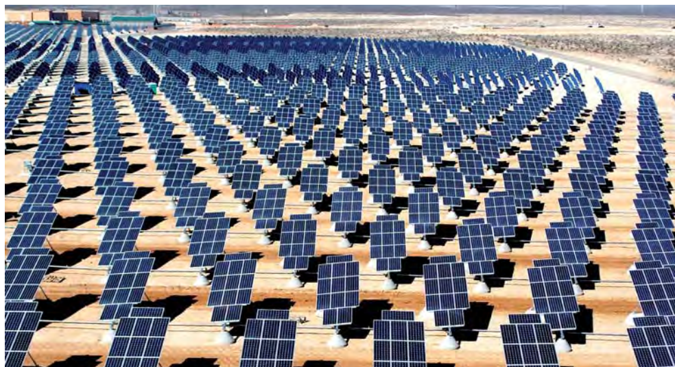
Figure 7.23 – 70,000 PV panels on the Nellis Air Force Base in Nevada, US generate 15MW of power
