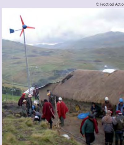
Figure 7.26 – One of 32 100W small wind turbines being installed in 'El Alumbre' in the north Andes of Peru. Three of the individuals shown were trained to install, operate and maintain the systems.
